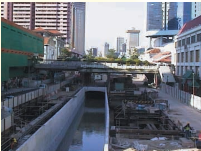
NEL Chinatown Station Ground shot showing the Reconstructed Eu Tong Sen Canal and the Underpinned Garden Bridge. Note the close proximity of existing shop houses and buildings on either side of the traffic deck that used to be Eu Tong Sen Street on the left and New Bridge Road on the right of the canal.
