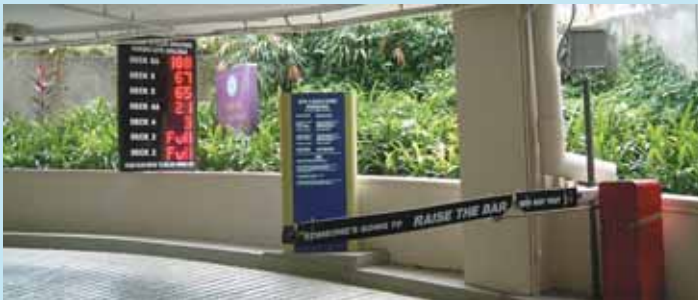
Integrated Electronic Payment System with Carpark Parking Guidance system
